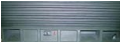
Grounded cast iron stator
